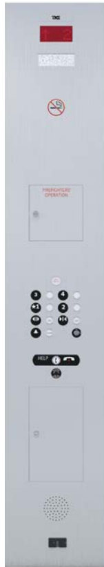
Car operating panel
