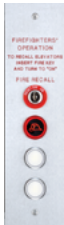
Intermediate hall station with fire services devices
